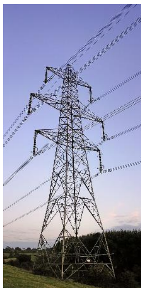
Figure B2.4: Lattice tower for 380-kV circuit
