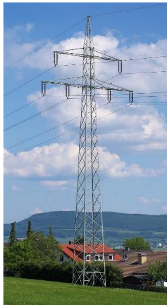
Figure B1.1: Typical structure for a transmission tower for two 110kV circuits
