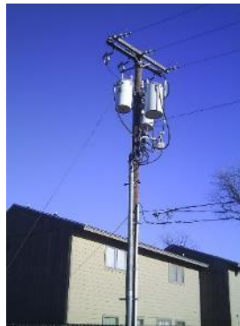
Figure B2.1: Wooden pylon for a mean voltage circuit in the USA
